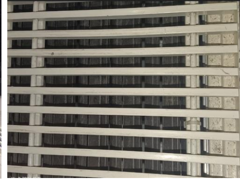
Supply Air grills closed
